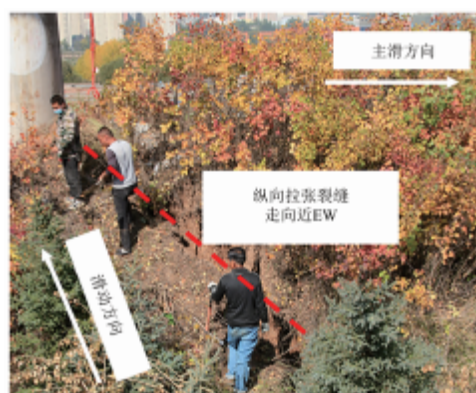
(a) 纵向拉张裂缝
